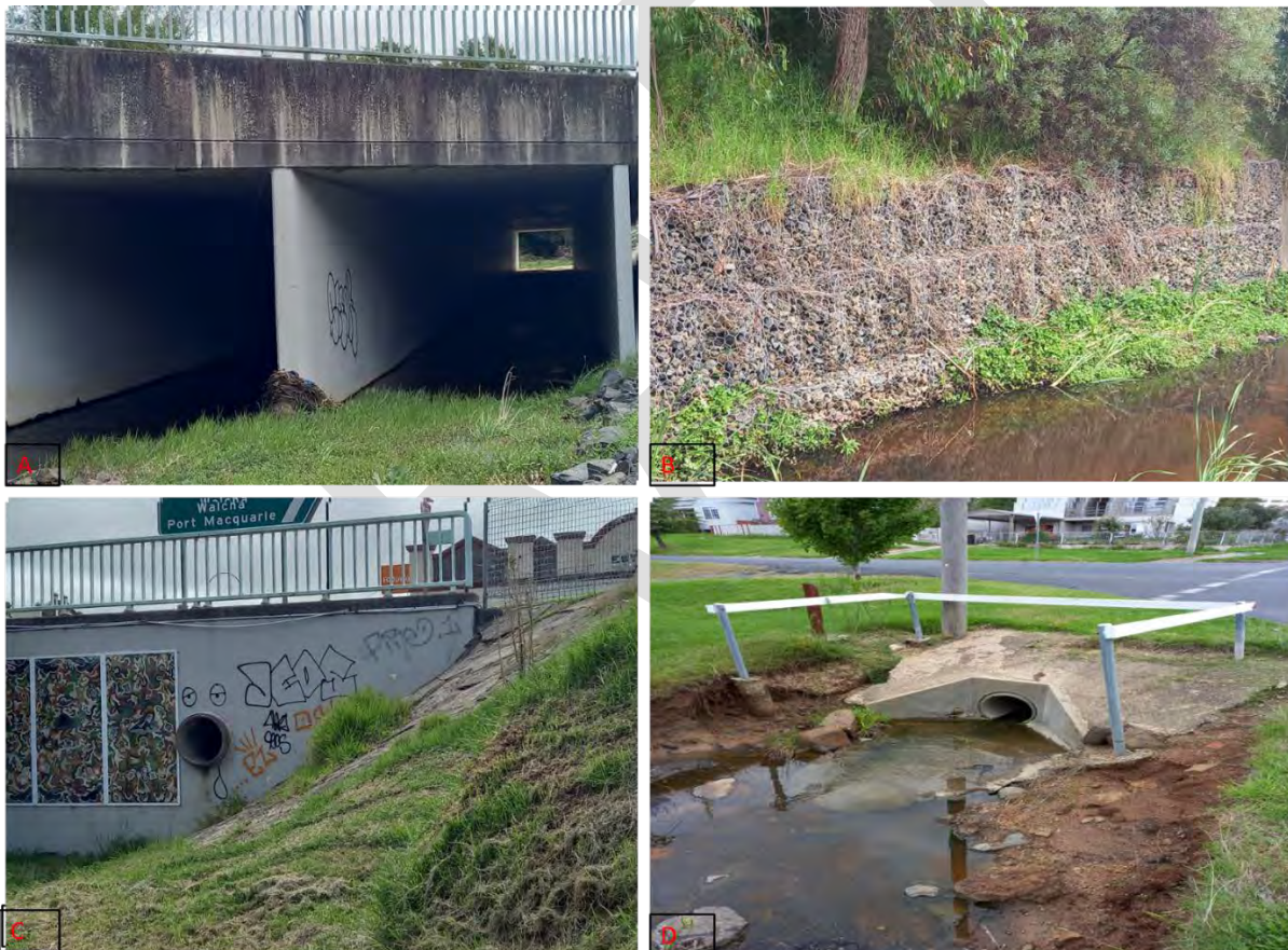
Figure 5.1: Examples of stormwater assets (A) Box culvert, (B) Waterway gabion protection (C) and (D) Pipes.
