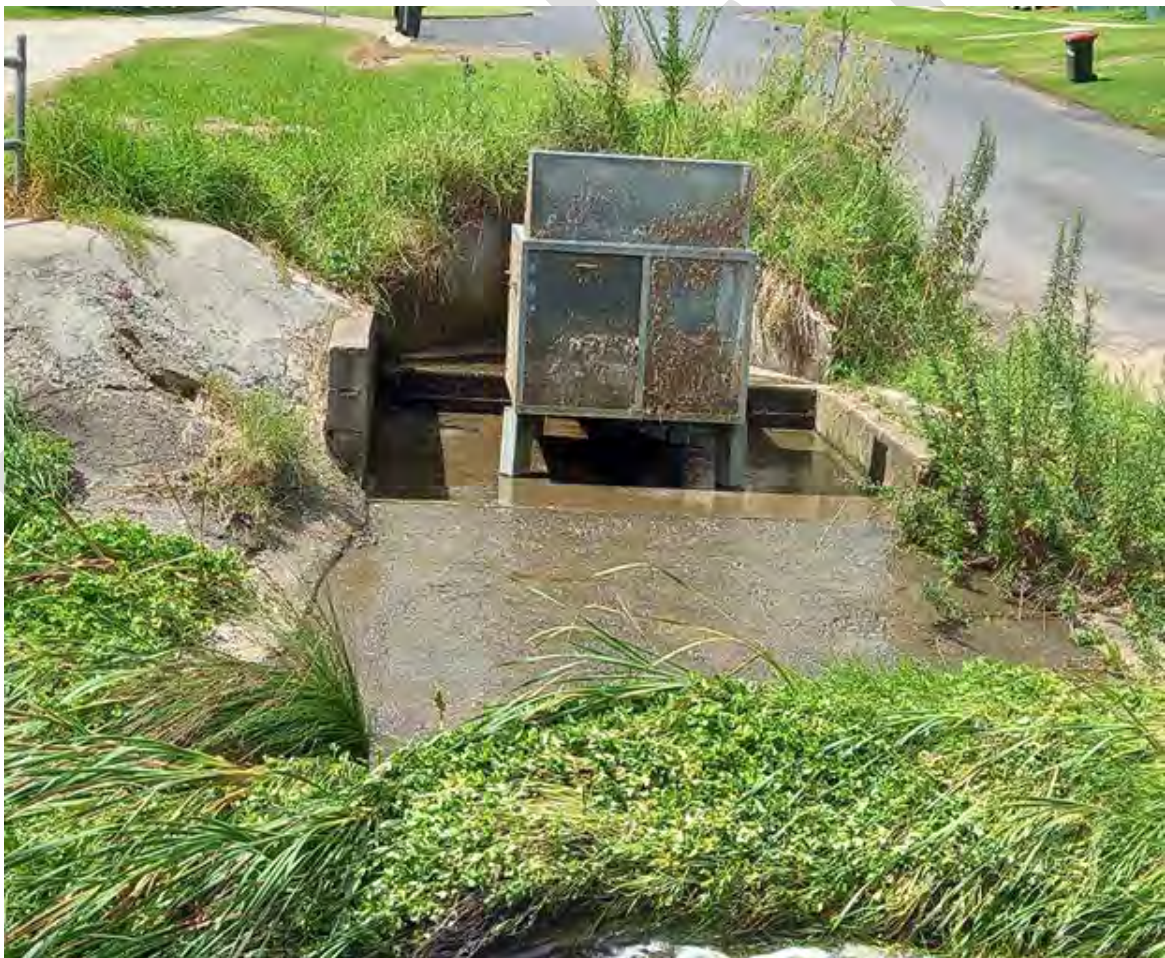
Figure 3.12.2: Gross Pollutant trap in “Excellent” condition
