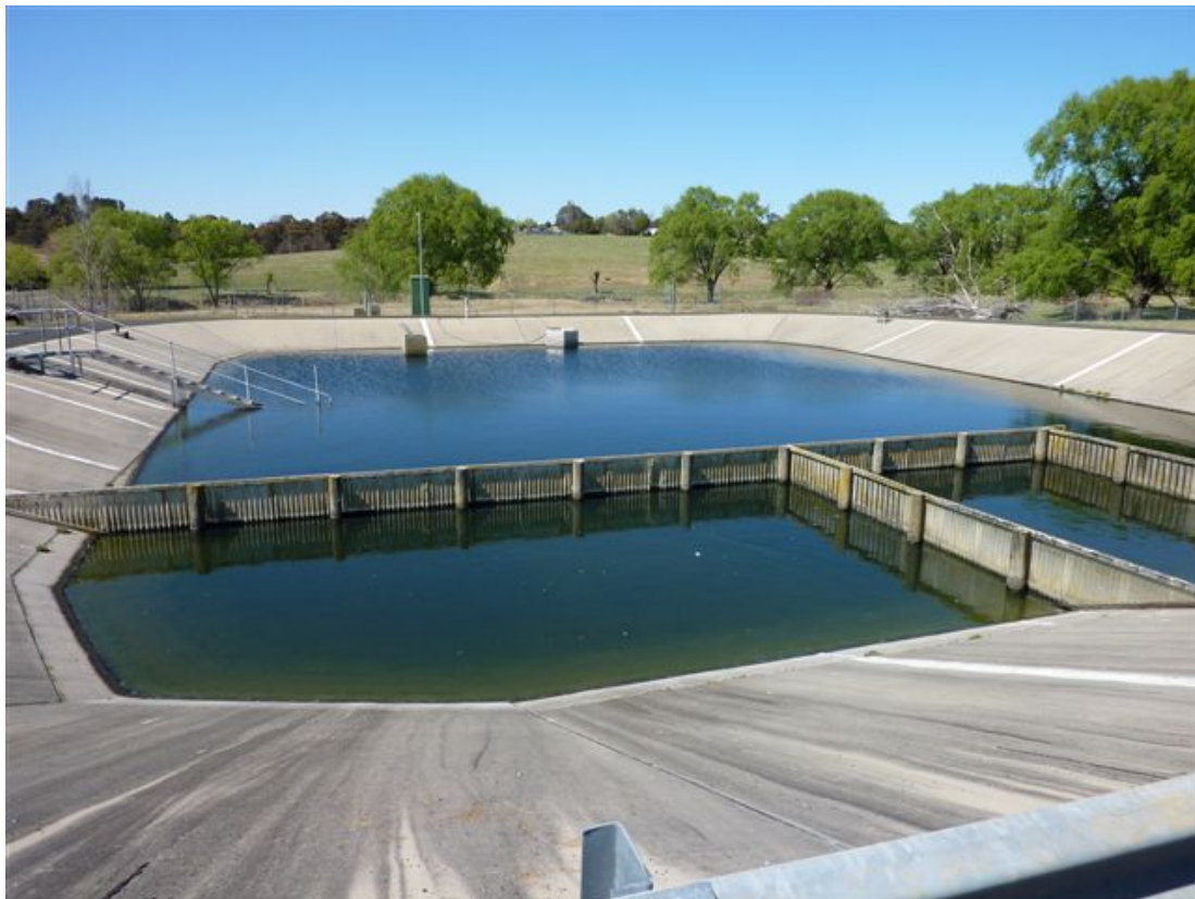
Figure 3.2 Catch Balance Tank.
