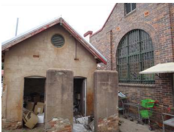
partially detached toilet block
