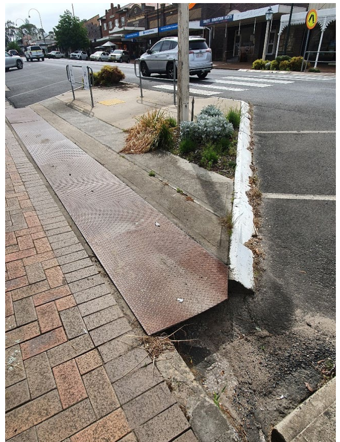
Image 5: Existing blister garden and pedestrian crosswalk in the Uralla CBD. Drainage cover between footpath and blister to be upgraded to improve accessibility and safety.
